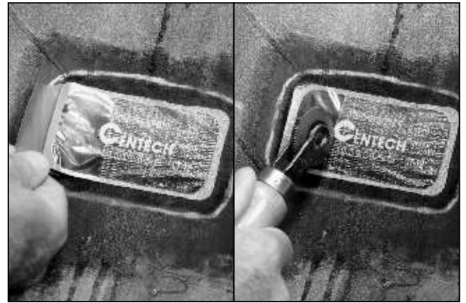
26 Remove the rest of the blue poly. Stitch the repair unit from the center to the outer edges.
